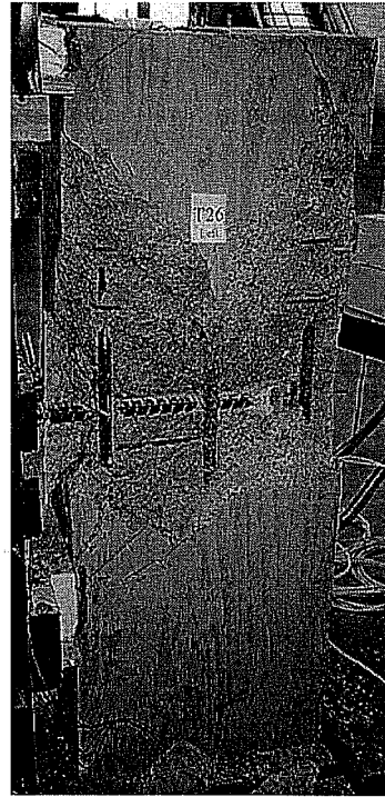
b) After spalled concrete fell off
